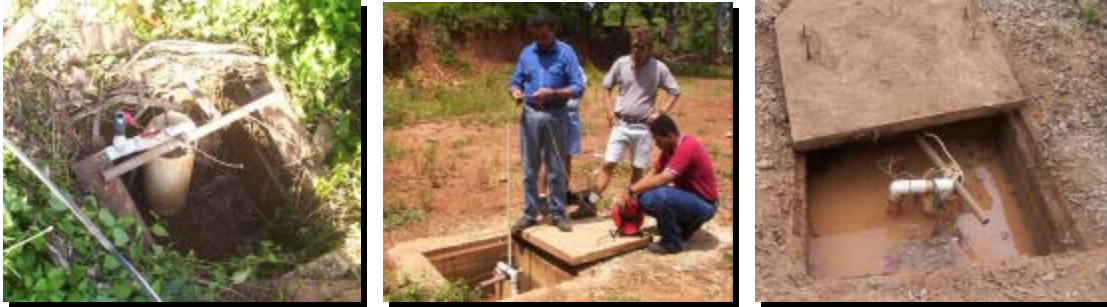
Figure 3-2. Utila Municipal Wells – MW 1, MW 2, and MW 3.
